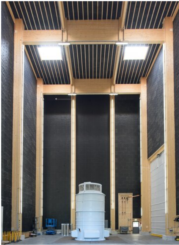
© Trench Austria GmbH
